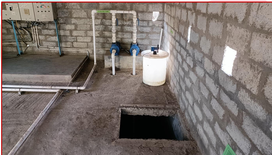
Filter Feed Tank (Capacity 40KL) and Filter Feed Pump
