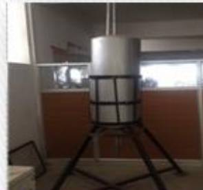
PCM Insulated Hot Water Storage Tank
